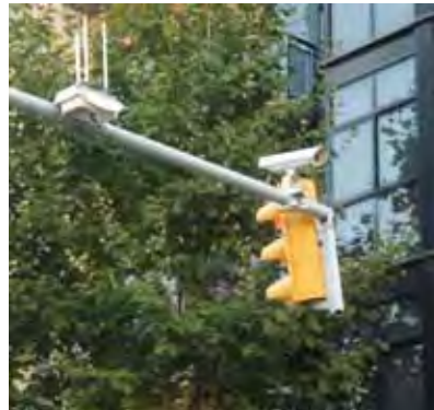
Traffic control cameras connected with optical fiber to the Public road headquarters made to control traffic in real time. It will be possible to increase or reduce the green frequency depending on the actual necessities
