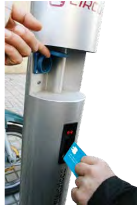
Charging points for electrical vehicles
